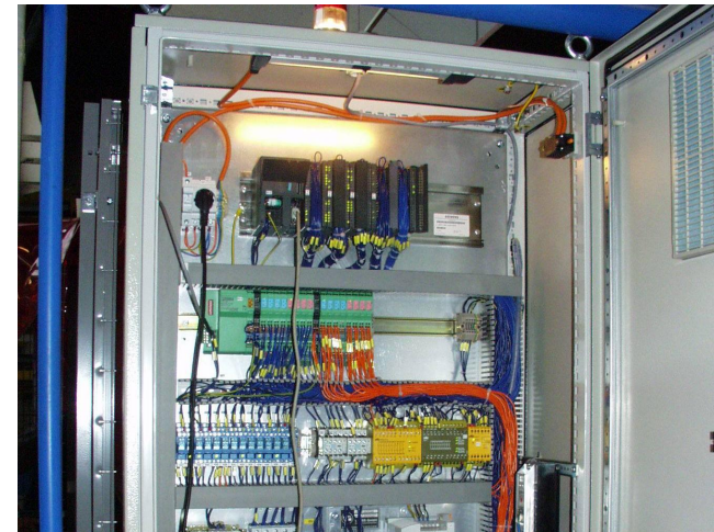
SIMATIC S7-314, InLine Module PHOENIX CONTACT, Safety Relays PILZ
